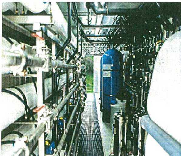
Imagine interior statia de epurare AST
